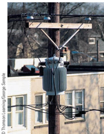
This transformer is smaller than the one in the opening photograph of this chapter. In addition, it is a step-down transformer. It drops the voltage from 4 000 V to 240 V for delivery to a group of residences.
